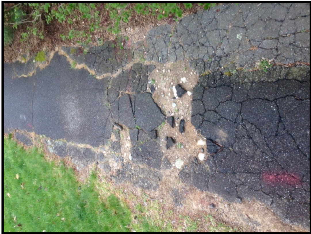
Photo of Teaberry Lane Sidewalk submitted with Sidewalk Petition.
